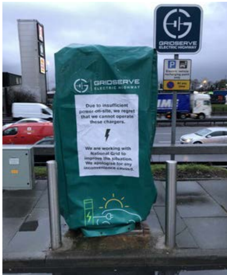
Broken EV charger
